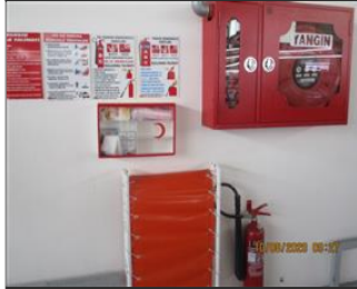
Photo of fire safety equipment FIRE HOSE AND FIRE EXTINGUISHER .JPG
