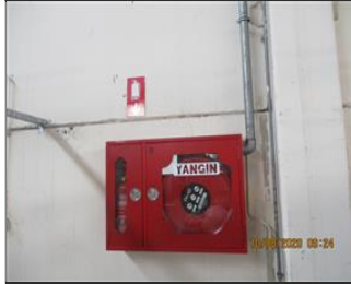
Photo of fire safety equipment FIRE HOSE .JPG
